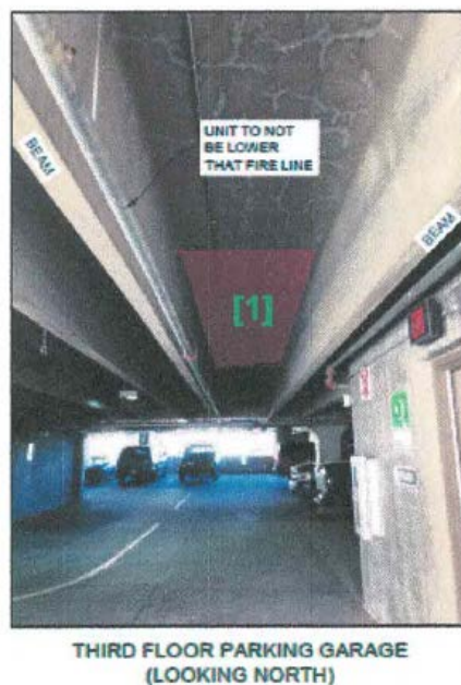
Figure 4: Proposed location for AT&T's HVAC equipment
