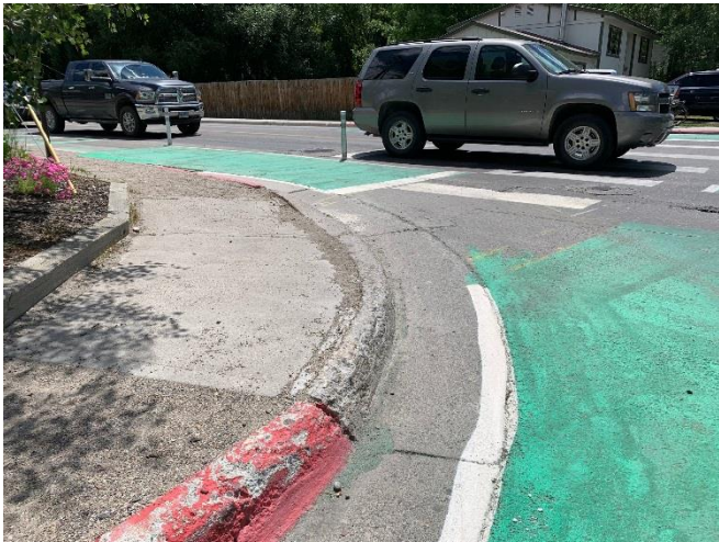
Figure 1 – Curb ramps do not comply with ADA
