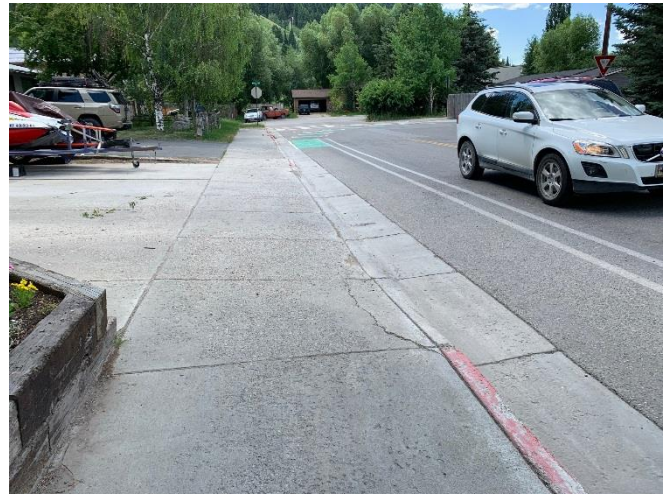
Figure 2 – Sidewalk cross slopes exceed 2%
