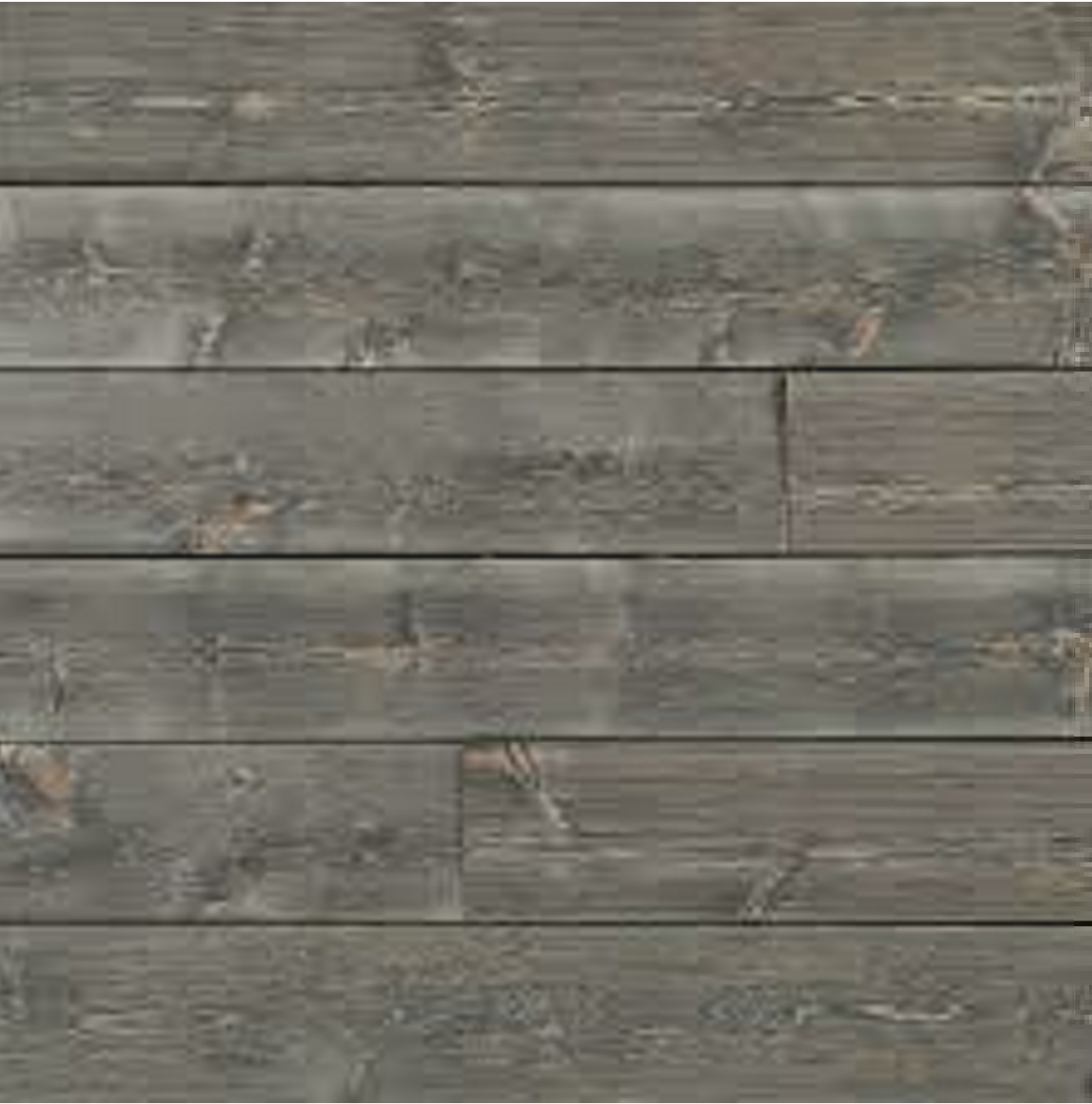
Weathered Wood Siding
