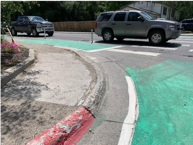
Figure 1 – Curb ramps do not comply with ADA
