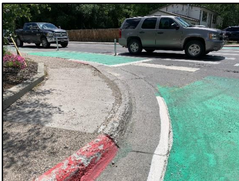
Non-compliant curb ramp
