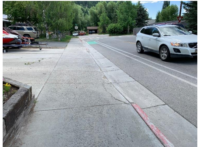
Figure 2 – Sidewalk cross slopes exceed 2%
