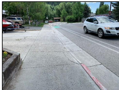
Non-compliant sidewalk cross slopes
