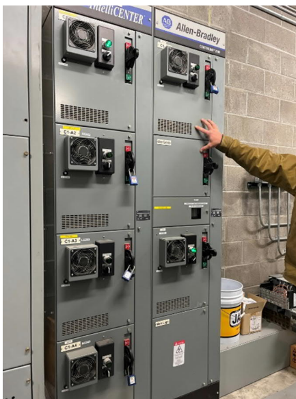
Photo 1.30. Influent Pumps SCADA
