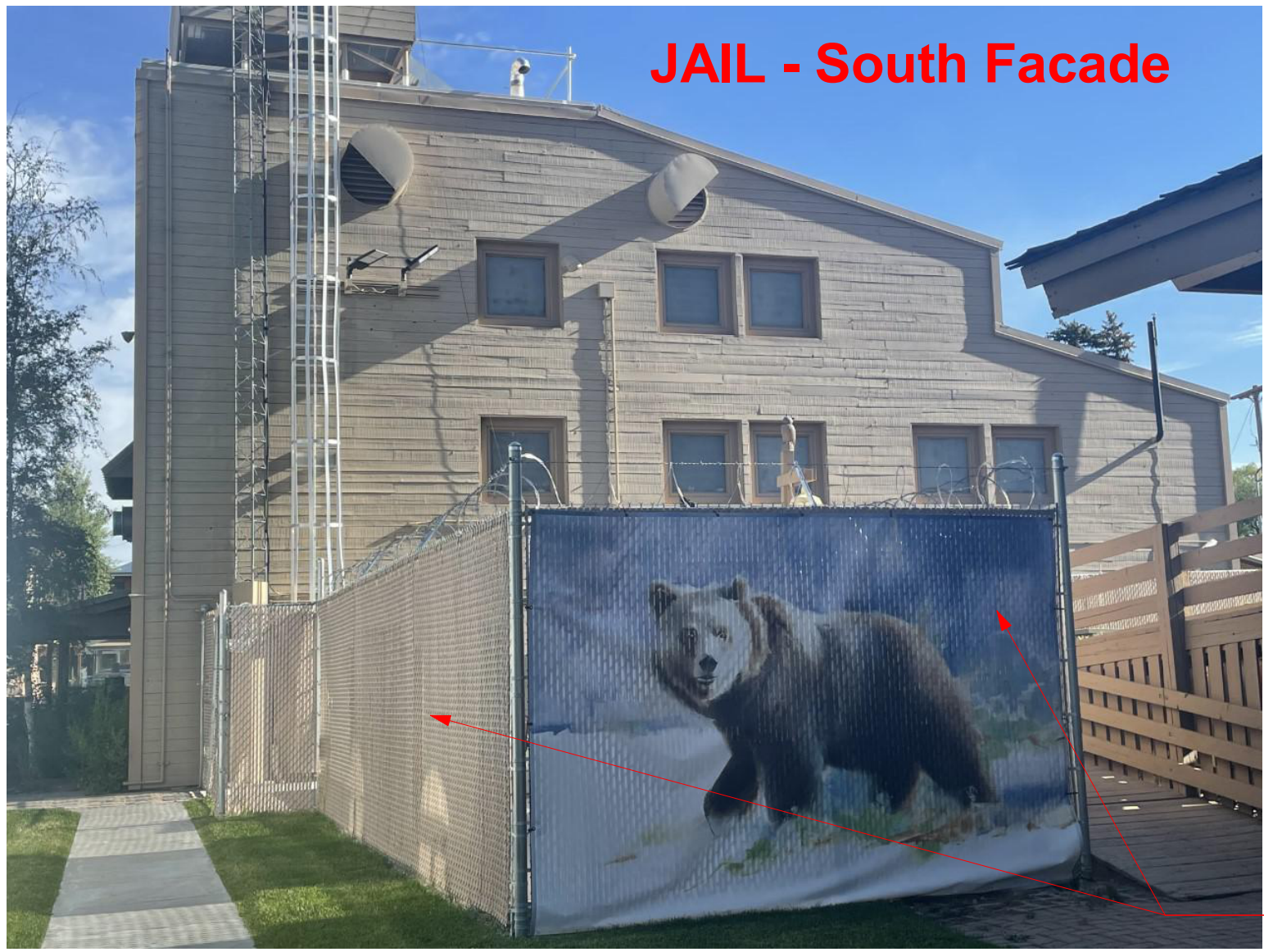
Existing Generator Enclosure
