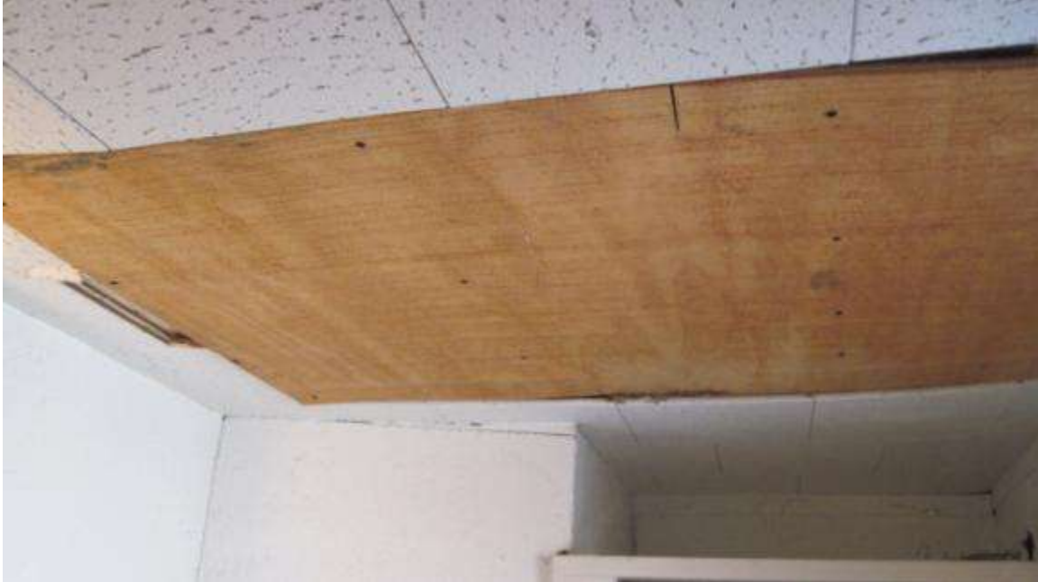
A view of some interior deferred maintenance.
