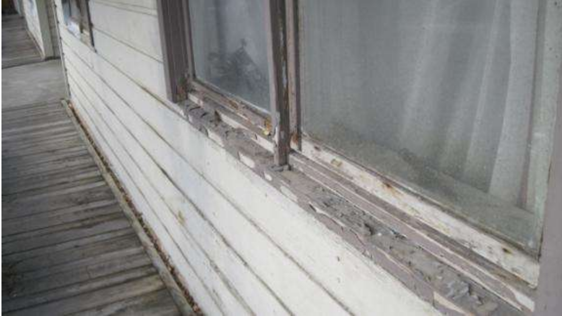
Views of some of the deferred maintenance
