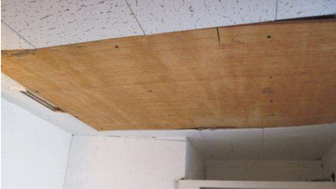
A view of some interior deferred maintenance.
