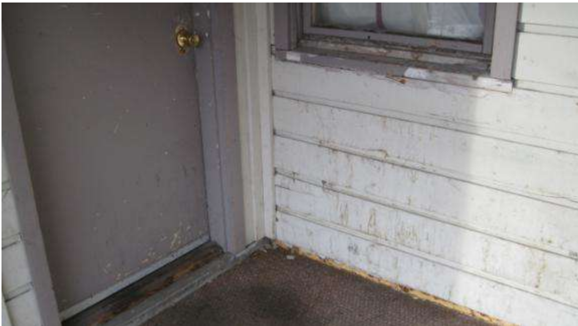
More views of deferred maintenance.
