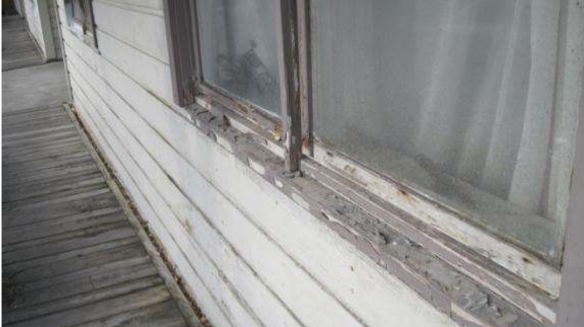
Views of some of the deferred maintenance
