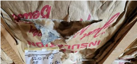
FIBERGLASS BATT INSULATION WITH PAPER WRAP ON NORTH HALF OF STRUCTURE
