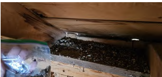
VERMICULITE INSULATION (VERM-1) IN ROOF OVERHANG BAY IN MIDDLE ROOM (<0.25% ACTINOLITE/TREMOLITE ASBESTOS)
