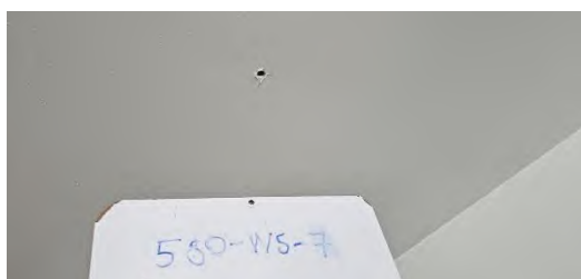
CEILING WALL SYSTEM SAMPLE IN LIVING ROOM (3.25% CHRYSOTILE ASBESTOS IN JOINT COMPOUND, 0.48% COMPOSITE)
