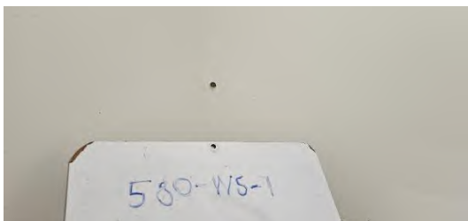
WALL SYSTEM SAMPLE IN LAUNDRY ROOM (2% CHRYSOTILE ASBESTOS IN JOINT COMPOUND, 0.21% COMPOSITE)
